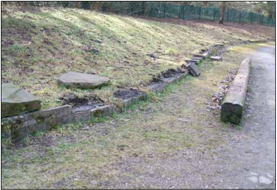
Damage to the low wall at Aberdulais Basin.
