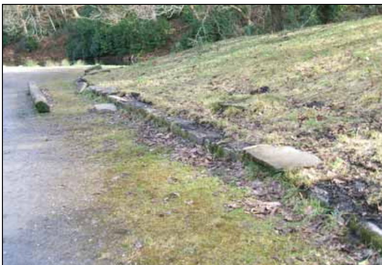
Damage to the low wall at Aberdulais Basin.
