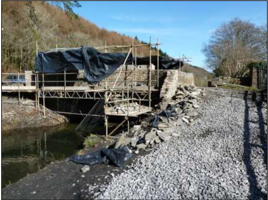
Work is nearly finished rebuilding the walls on the bridge across the Neath Canal into Ynysarwed Farm.
